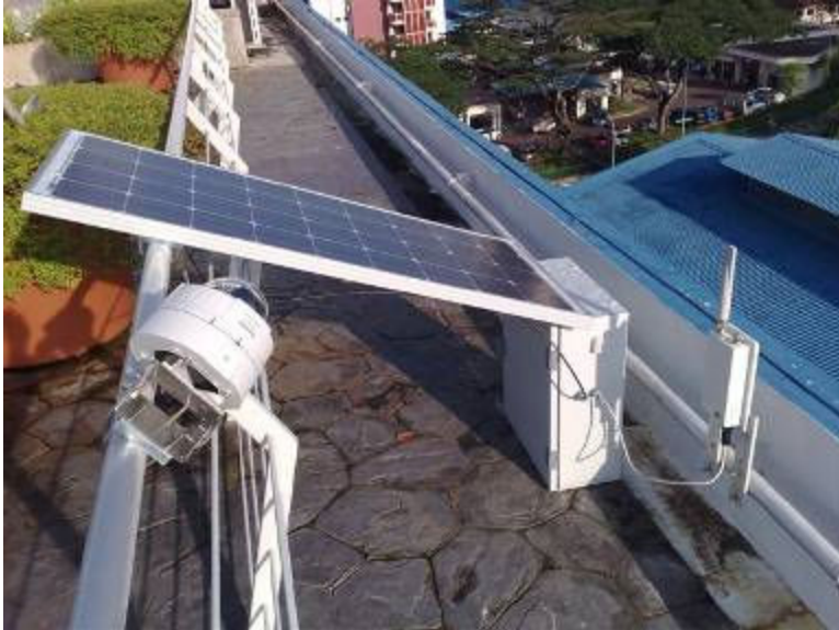
Setup of Solar Powered Wireless Surveillance
